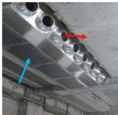
Air dryer system
